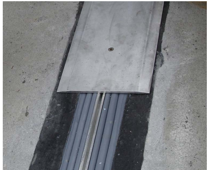
SJS-FR SYSTEM installed with EMCRETE elastomeric nosing material in blockouts on each side of joint gap.
