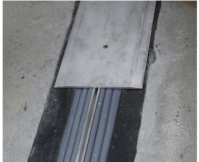
SJS-FR SYSTEM installed with EMSEAL elastomeric nosing material in blockouts on each side of joint gap.
