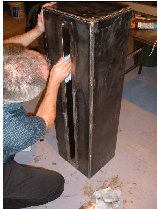
Figure A2 – Cleaning Inside of Fixture Gap with Xylene Prior to Installation of Expansion Joint
